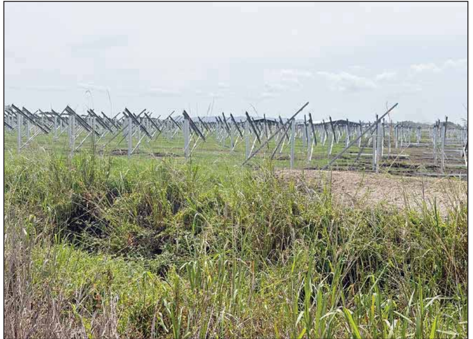
Rows and rows of stands for solar panels alongside McCathie Rd. as Meridians Energy's Ruakākā Solar Farm takes shape
