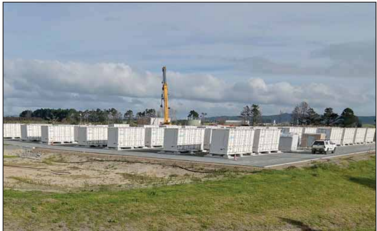
The Battery Storage System nearing completion at the corner of Marsden Point Rd. and Rama Rd. in Marsden Point
