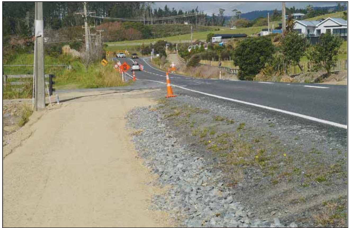
The new section of the Waipu to Waipu Cove cycle and walkway
