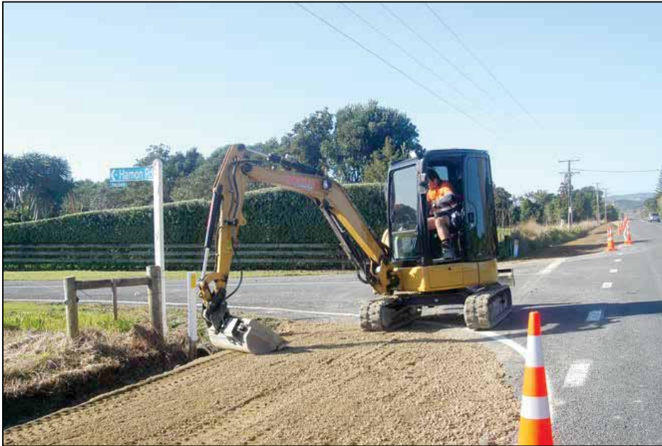
Paul Cowpland finished the trail section to the Waipu Cemetery on Wednesday 14 August 2024
