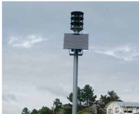
A new tsunami siren in Ruakākā Village
