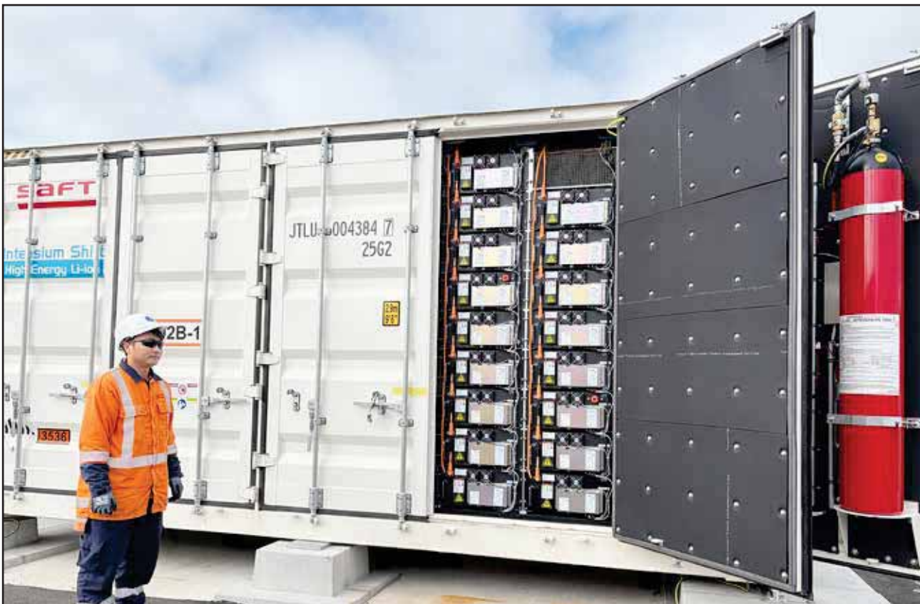
Field service engineer Minh Nguyen opens a door on one of the 80 containers to reveal stacks of battery modules. The batteries were built in China for French Company Saft. Mr Nguyen is employed by Saft to oversee the system. He works alongside electrical engineers from McKay Electrical who he said have impressed him as very professional.
